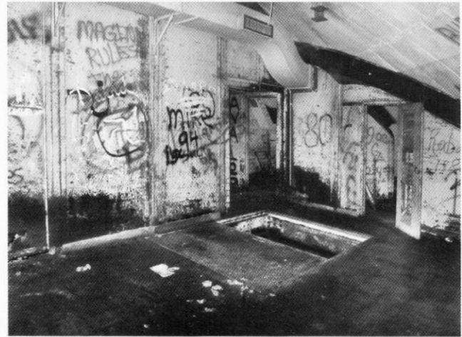
The interior of the MDF room showing the 'hole of doom', the open equipment access hatch to the lower level. The mindless graffiti with which this site was liberally daubed can also be seen
